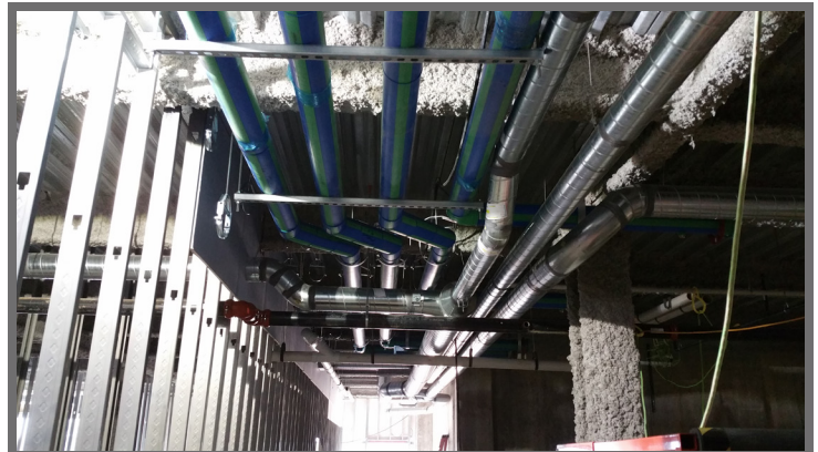
PPR piping and spiral ductwork in the mechanical room.
